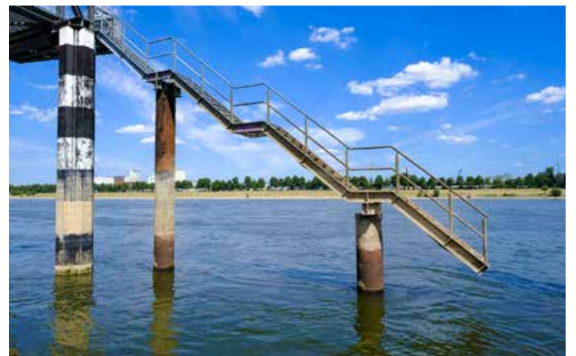
Oxidation on the stairs of a pontoon at the Rhine River illustrates just how far the water level has fallen. (Image: Thierry Monasse/Getty Images)
